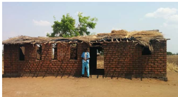
Figure 3: A HSA stands in front of a Village Clinic structure that was constructed by the community
