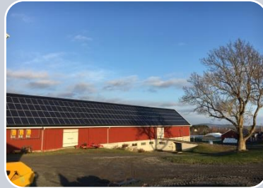
Commercial PV plants & Smart buildings
