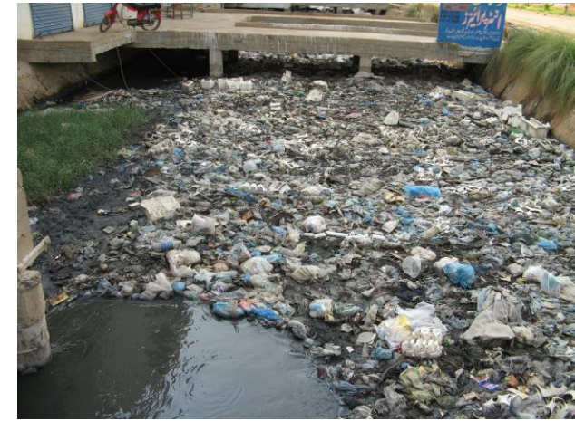
Korangi Drain Canals
