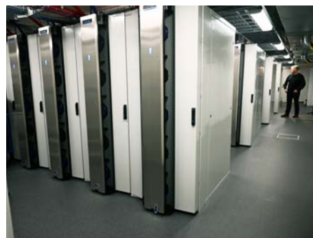
A state-of-the-art server room.
