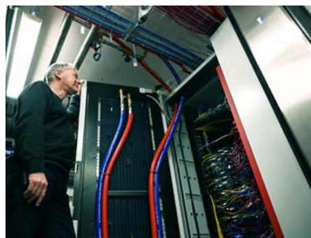
Senior Engineer Torben Leifsen shows us what's inside the racks.
